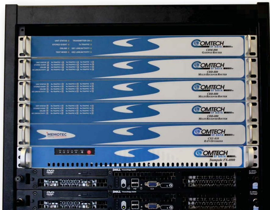
Advanced VSAT Solution installation with CXU 810
