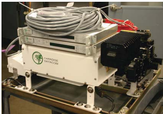
125W Ku-Band 1:1 Phase Combined SSPB System with FPRC-1100 Controller and RCP2-1100 Controller for L-Band redundancy
