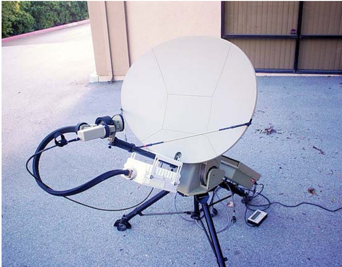
Figure 3.2 IBUC 2 Field Installation
