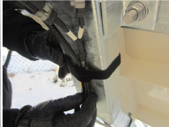
Polarization Motor and Inclinometer
